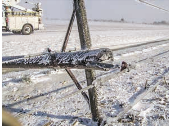
PHOTOS COURTESY OF SAFELECTRICITY.ORG
